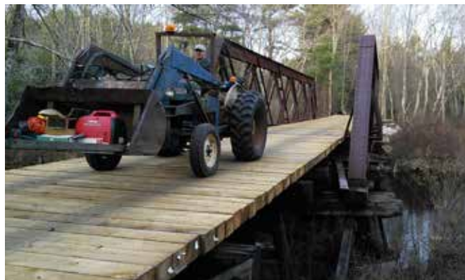
Mark with his tractor at the pony truss after finishing the decking repairs.
