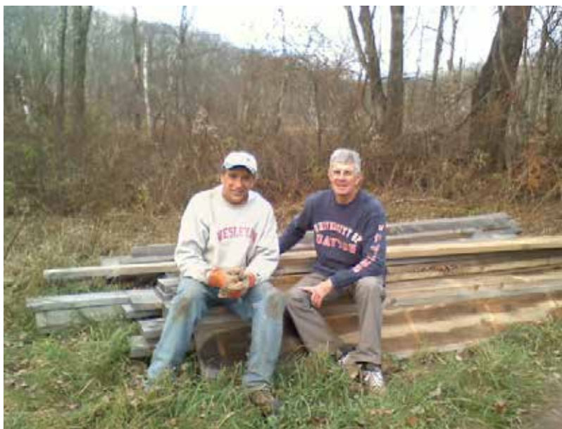
Rick Romano and Neil Dawson after a full day of clearing trail and installing boardwalk resting on more planking for the trail network.
